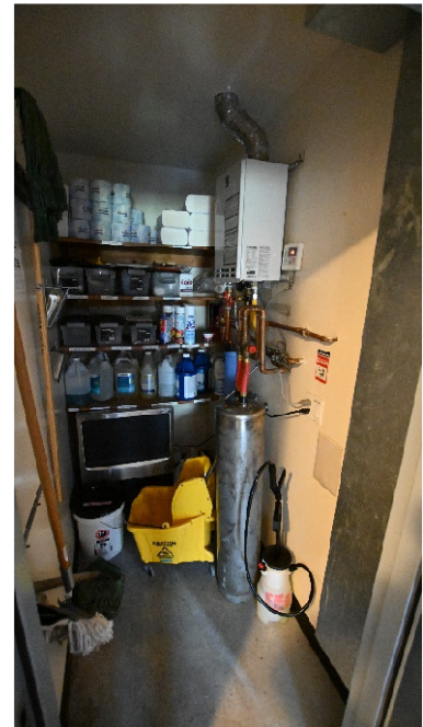
Under-sized Instant Wall-Mounted Water Heater
